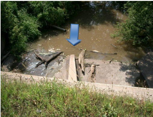
Debris at inlet; no sedimentation
