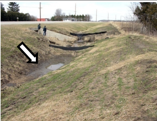
Side view (left bank) showing the new work. Local scour depressions evident just upstream the silt fences. (see white arrow)
