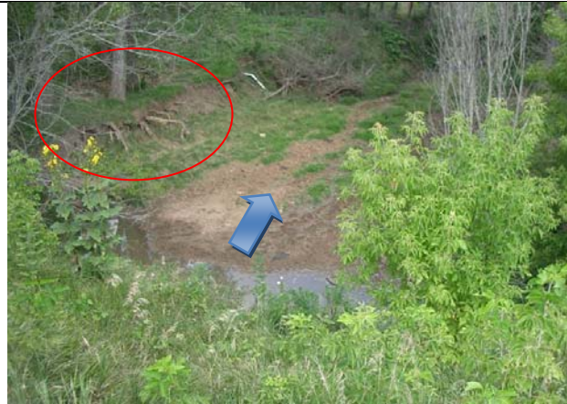
The red circle shows serious bank erosion on the left bank downstream the culvert
