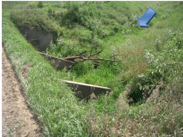
The channel enters the culvert with a large angle. Arrow indicates the thalweg of the channel.
