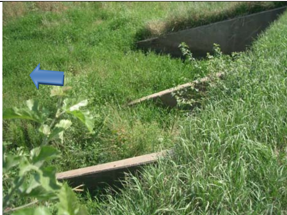
Sedimentation is also serious downstream of the culvert.
