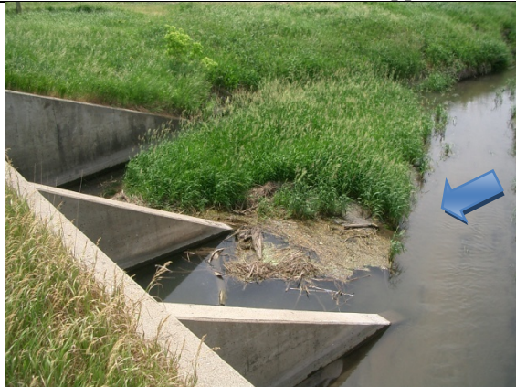
A sediment bar at culvert entrance
