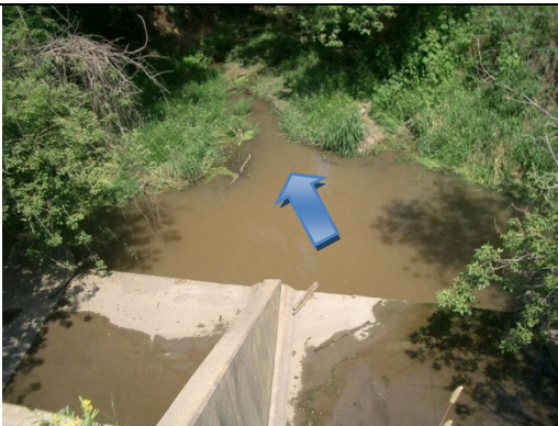
Outlet invert is higher than the channel bed. The downstream channel is not well aligned with the culvert
