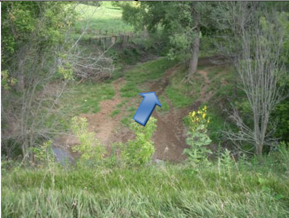
The downstream channel is not well aligned with the culvert
