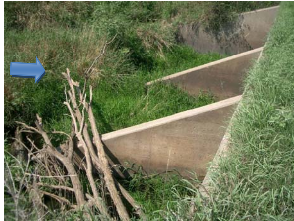
Serious sediment and debris accumulation. Sediment accumulation in three barrels.
