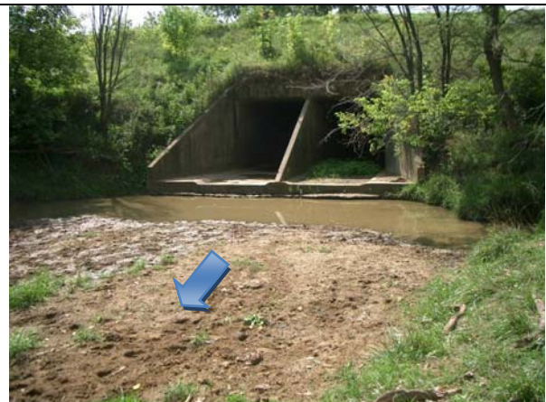
A scour hole at the culvert exit.
