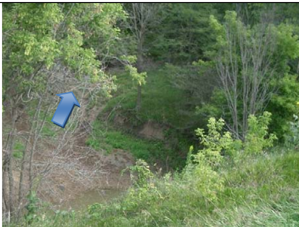
View of the right bank downstream the culvert. Bank erosion is also on the right bank.
