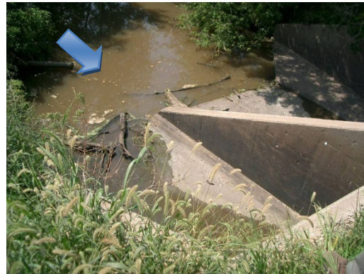
Inlet invert is higher than the channel bed
